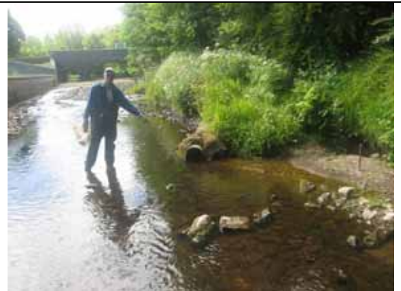
Site 2. Galey River. Downstream of Athea Bridge for c.150m. Generally unsuitable habitat due to heavy siltation and filamentous algal growth. No evidence of mussels. View of raw sewage entering river from pipe.
